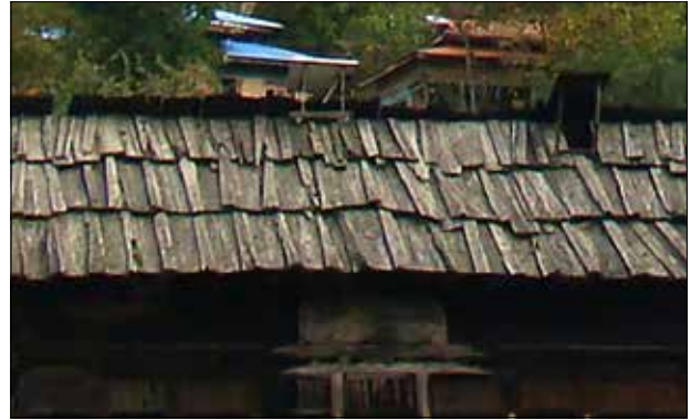
Figure 22. Birch bark, a waterproof coverage for gabled roofs, also water conductors for snow and rain (Photograph: Authors).
