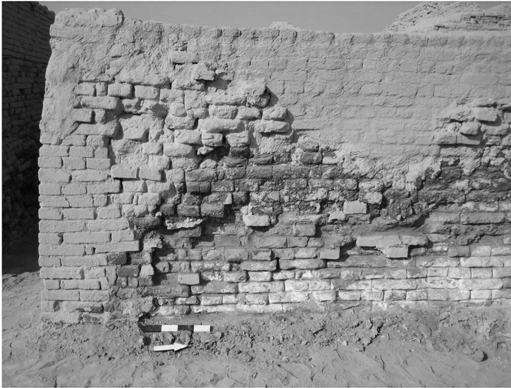
Figure 3: Moenjodaro, Soluble salts attack at main street, DK-G area.
