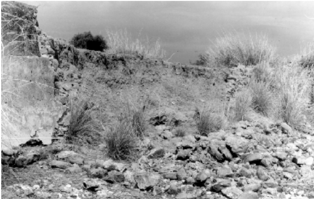
Pl. 5b. Karak (Sultan Shāh Nika): Reservoir broken wall section showing different phases of construction.
