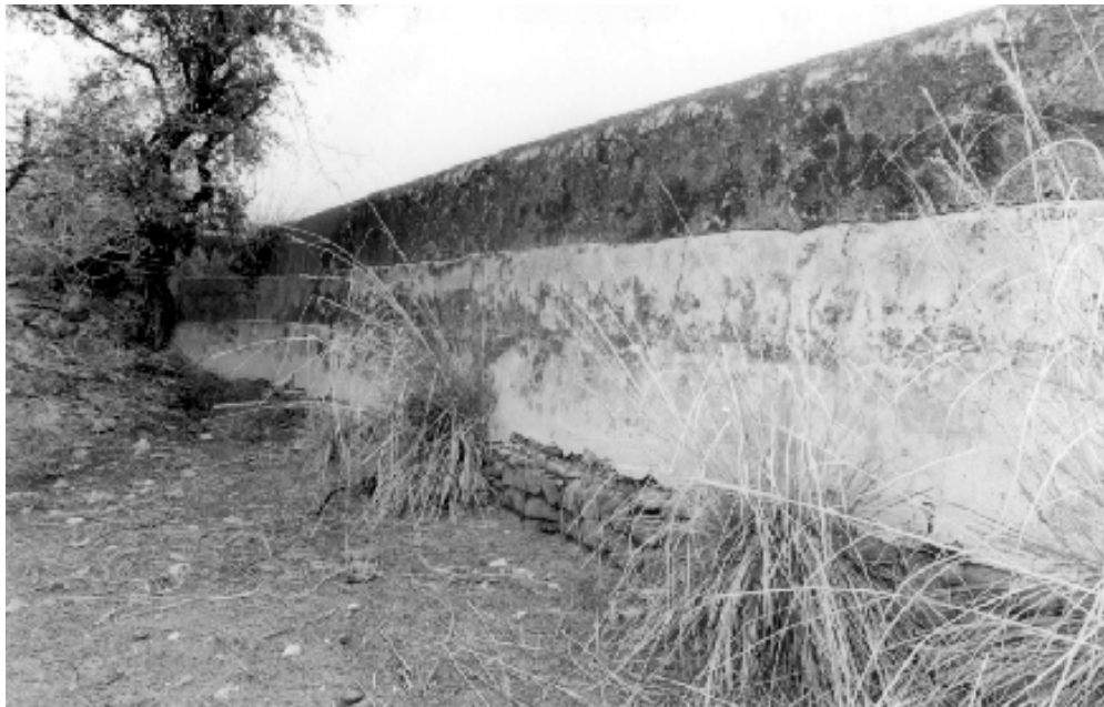
Pl. 5a. Karak (Sultan Shāh Nika): An eight feet high wall of the reservoir showing different phases of construction.
