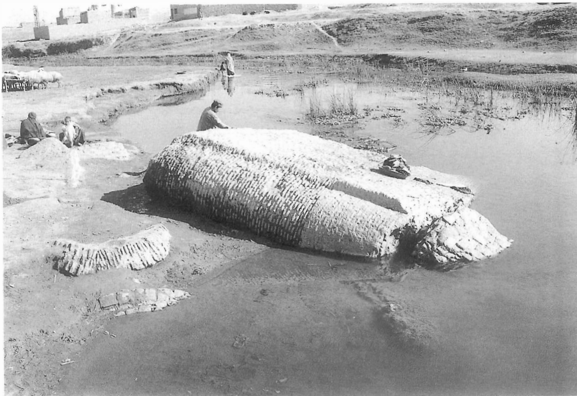
Pl. 5: Zinda'i Bridge: Fallen pier.
