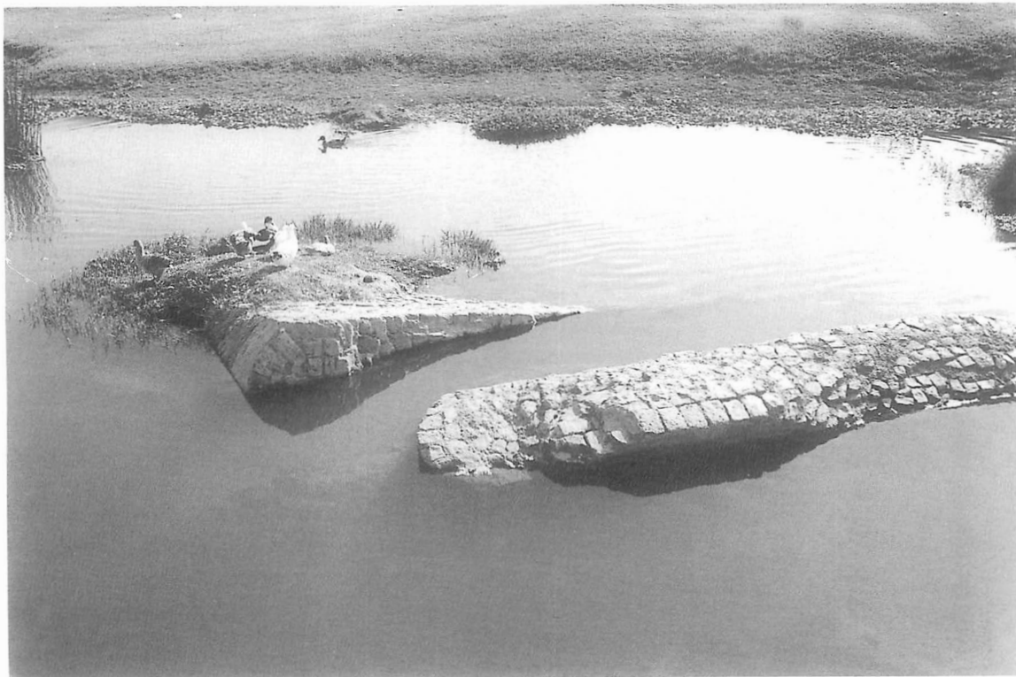
Pl. 6: Zinda'i Bridge: Another pier fallen in the stream water.
