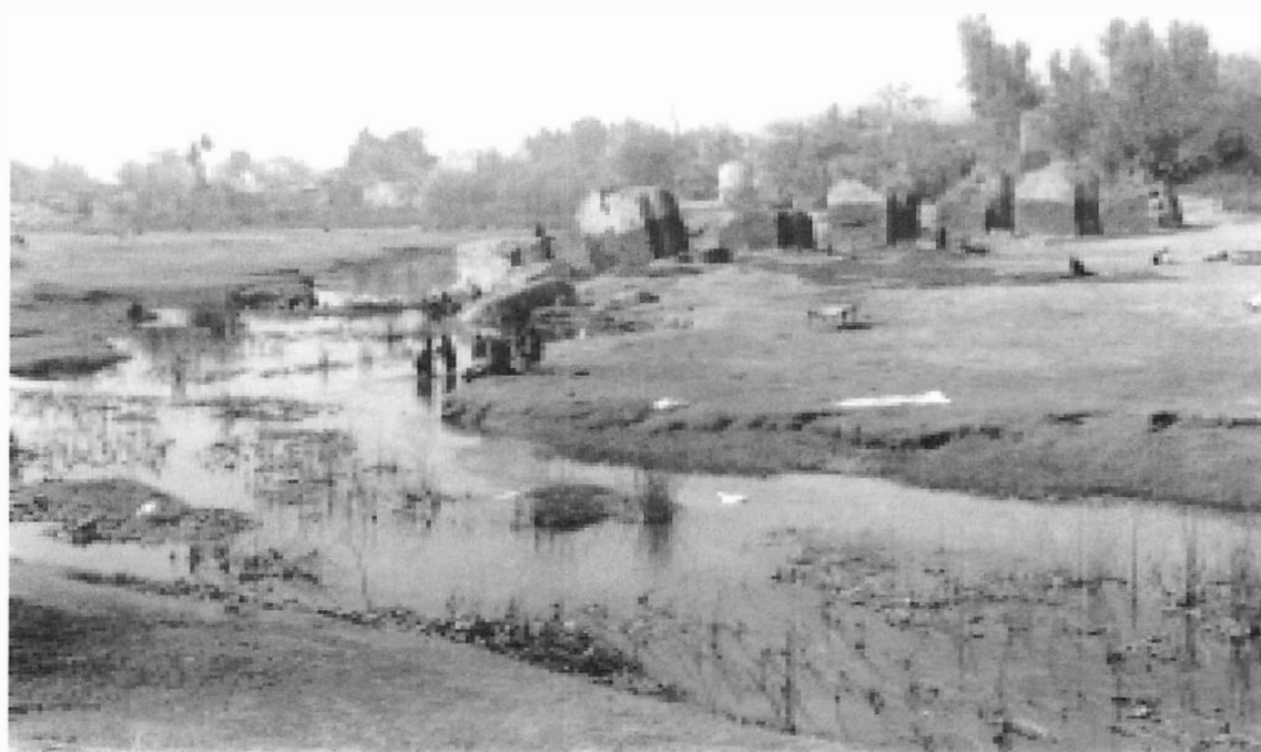
Pl. 4: Zinda'i Bridge: View of the bridge from the north with the Zinda'i stream in the foreground.
