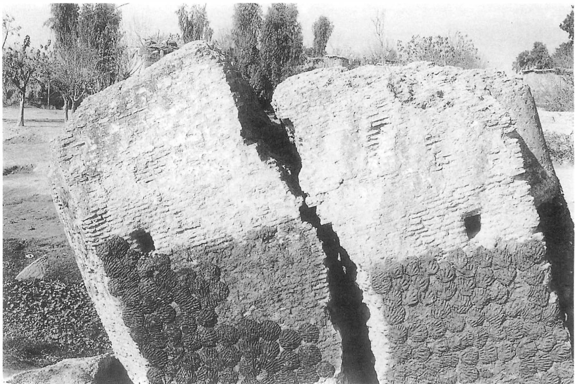
Pl. 8: Zinda'i Bridge: Close up of the pier which is at the threshold of collapse.
