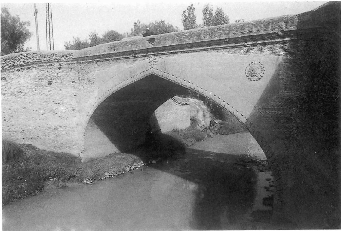
Pl. 2: Chamkani: A small bridge on the Bārā stream near modern G.T. Road.
