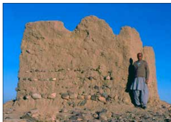
Figure 5. Farid Khan beside an abandoned building in the Jani Khel, Bannu District. The original mud plaster finish has fallen off in places, revealing courses of river-rolled pebbles and cobbles embedded in mud mortar. Observations such as this helped explain why the surfaces of many ancient sites are littered with river-rolled stones (as discussed in the text), (Photograph by the author)
