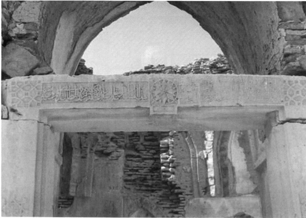
Fig. 5. Tomb of the sister of Jam Fateh Khan: Arabic inscription in thulth character on the outer lintel of the eastern entrance
