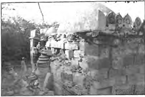
Photo 3. A historical mosque near Nagar Parkar built in Mughal times suffered partial collapse in response to ground shaking.
