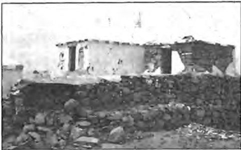
Photo 4. Hindu temples near Nagar Parkar showing partial collapse in response to ground shaking.
