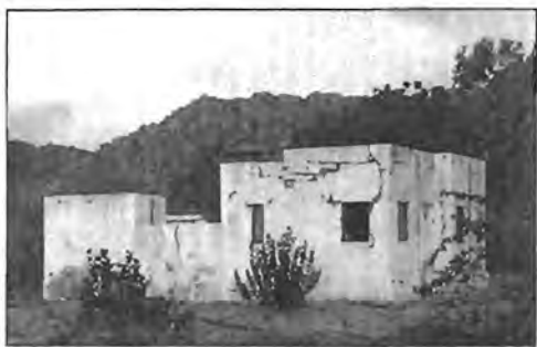
Photo 5. A school building at Nagar Parkar developing extensive cracks in response to ground shaking. Such relatively modern governmental masonry buildings experienced more damage than privately owned older masonry buildings, due to poor quality building material and workmanship.
