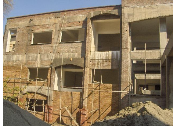
Fig. 1. Administration Block, NWFP University of Engineering and Technology, Peshawar (a new 4-story RC frame building).
