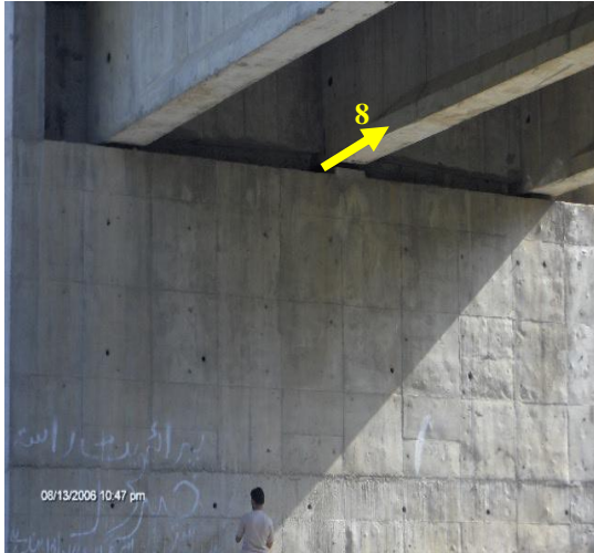
Fig. 8. Location of 1 sensor at abutment.
